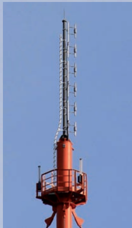
VHF DAB+ "Raichberg" transmitting antenna
